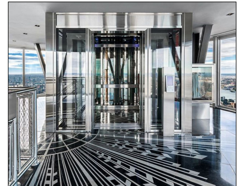
The new custom-made Gen2® glass “mast car” elevator installed by Otis in 2019 now carries visitors to the Empire State Building’s reimaged 102nd floor Observatory. The installation capped a yearslong modernization of the New York landmark — among the largest and most complex projects in Otis’ history.
